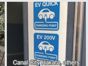
Canal City Hakata, others EV charging station
